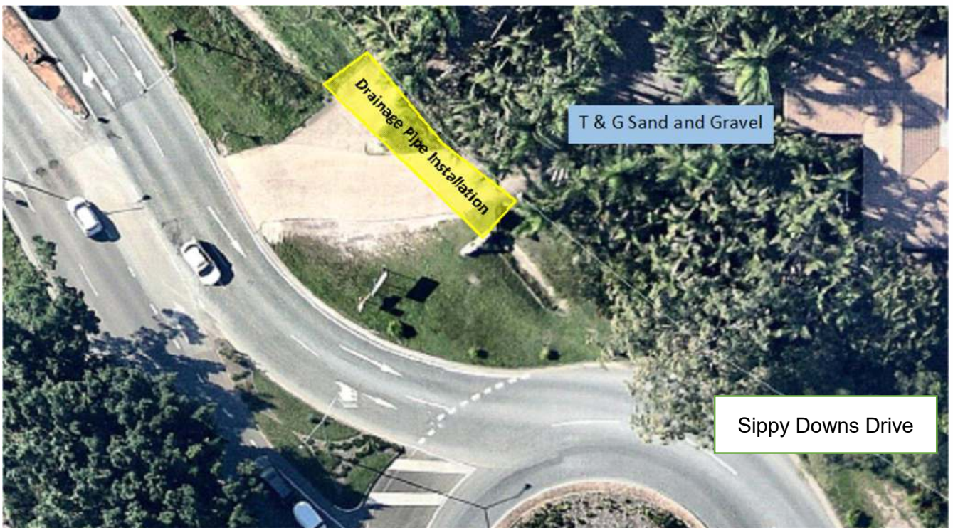
Figure 1. Temporary changes to traffic conditions – Installation of Stormwater drainage pipes across existing T & G Sand and Gravel driveways.
